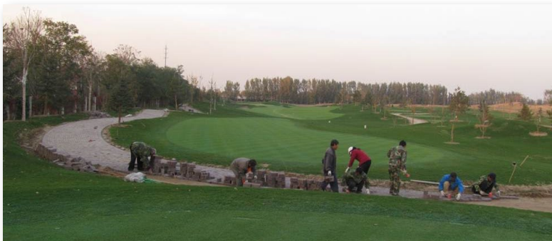
Top Photo: Bunker lining installation at Tianjin Pearl Beach International Country Club Bottom Photo: With grassing completed on parts of the course, the crew moves on to cart path construction at Nicklaus Club - Beijing
